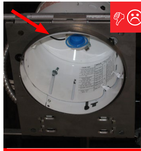
C. No gasket installed.
