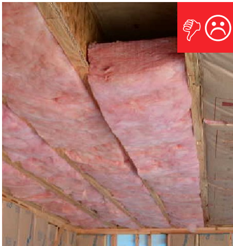
C. Insulation is misaligned with floor above.
