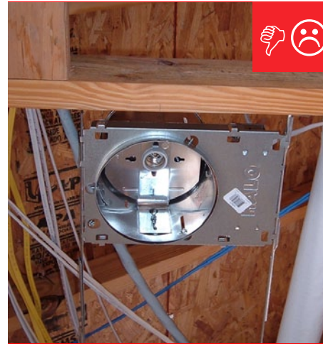
A. Non ICAT recessed light installed.
