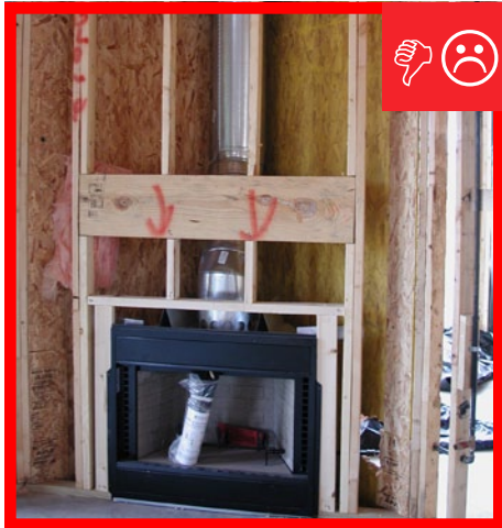
A. No insulation installed behind fireplace.
