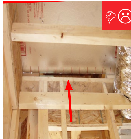
B. Seams of air barrier not sealed.
