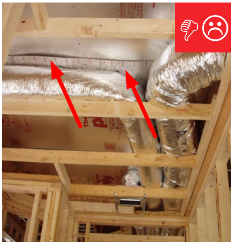
B. Seams of air barrier not sealed.
