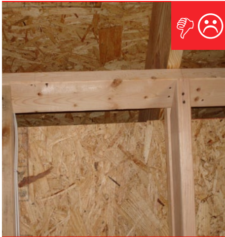
A. Air barrier is not continuous.
