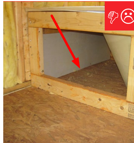
C. Air barrier not sealed.
