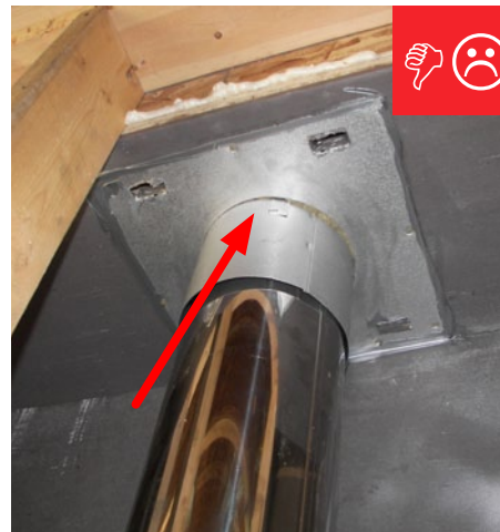
C. Vent sleeve not completely sealed.
