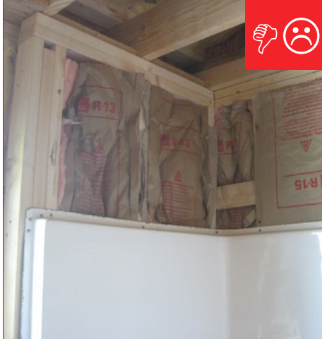
A. Insulation has compression and misalignment.
