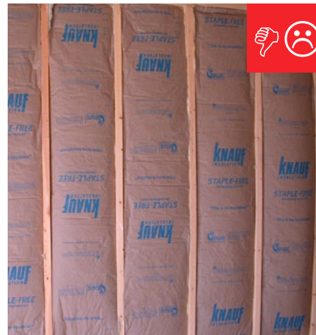
C. Insulation is misaligned.
