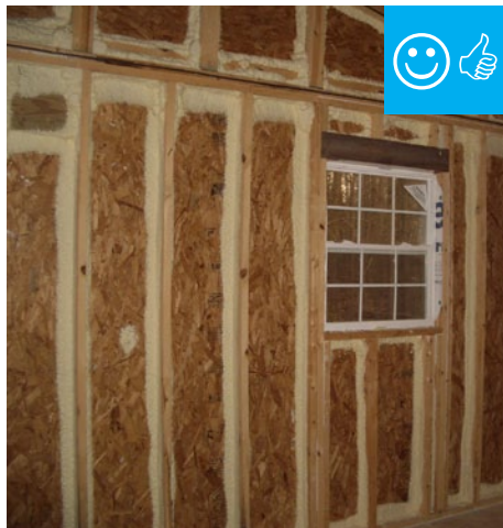
Air barrier is air sealed.
