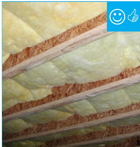
Insulation is in contact with floor above.
