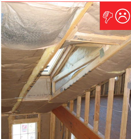
C. Insulation is misaligned with air barrier.
