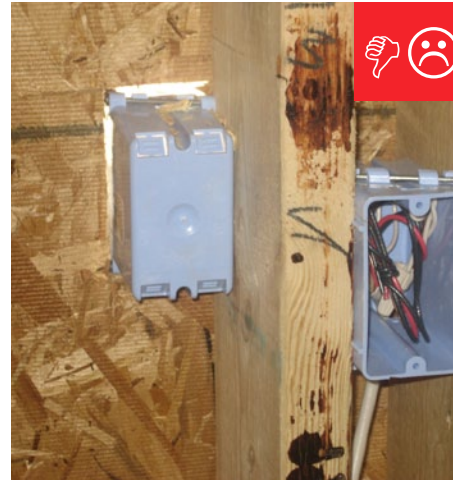
B. Electrical box not air sealed.
